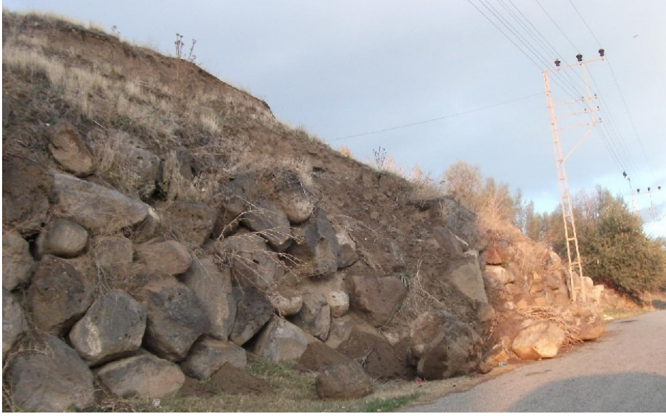
Figure 7.19. Toppled wall of Urartu castle in Çelebibağ village (Erciş).
