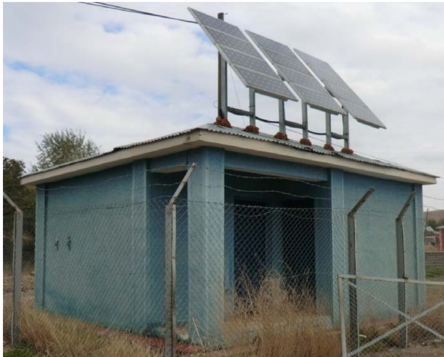
Figure 9.11. A view of pumping facility in Alaköy.
