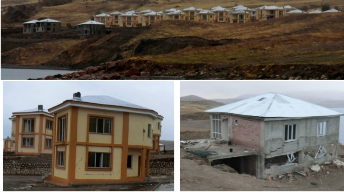
Figure 7.6. Damaged low story villa-type buildings constructed on sloping ground along the shore Van Lake.
