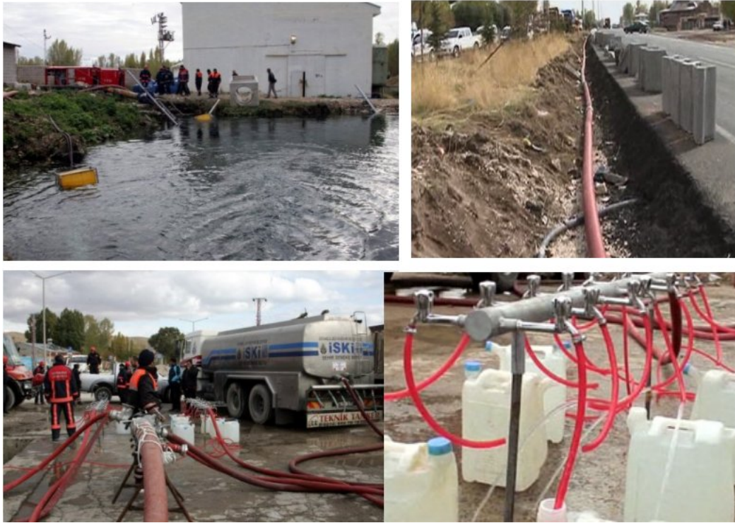
Figure 9.10. Temporary water supply system set up by İstanbul Municipality Water Department .
