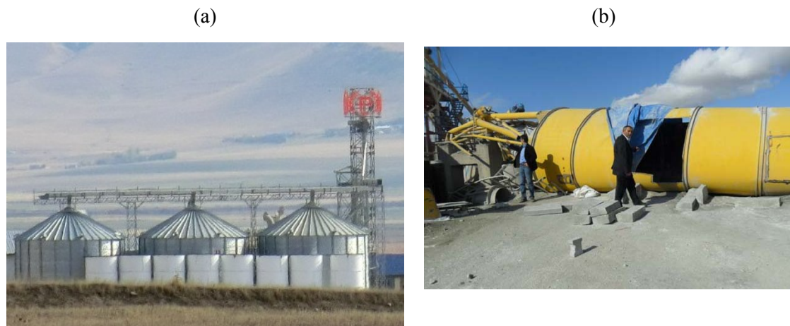
Figure 7.11. (a) Non-damaged silos in Van and (b) collapsed cement silo in the Van Industrial complex (KOERI, 2011).
