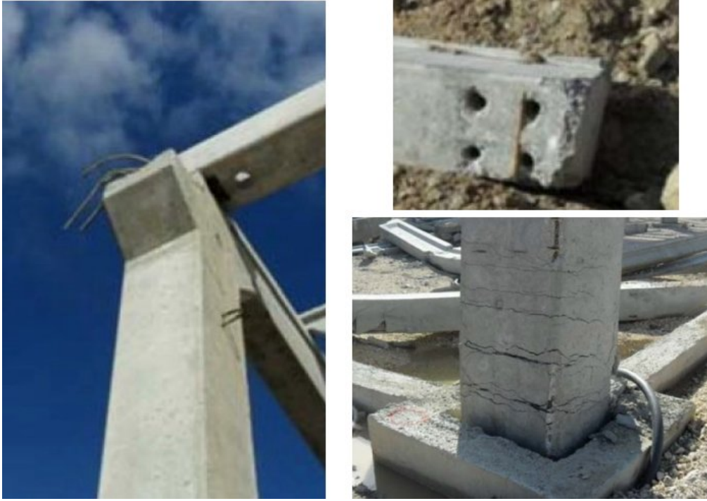
Figure 7.15. The details of poorly constructed beam-column connection of the pre-cast structure shown in Figure 7.14 (pictures arranged from KOERI (2011)).
