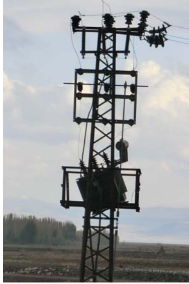
Figure 9.6. Dislodged transformer on a utility pole in Erciş.
