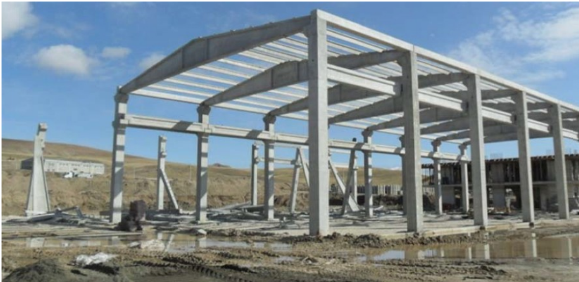
Figure 7.14. A view of heavily damaged pre-cast reinforced concrete structure in Van Industrial Complex (from KOERI, 2011).
