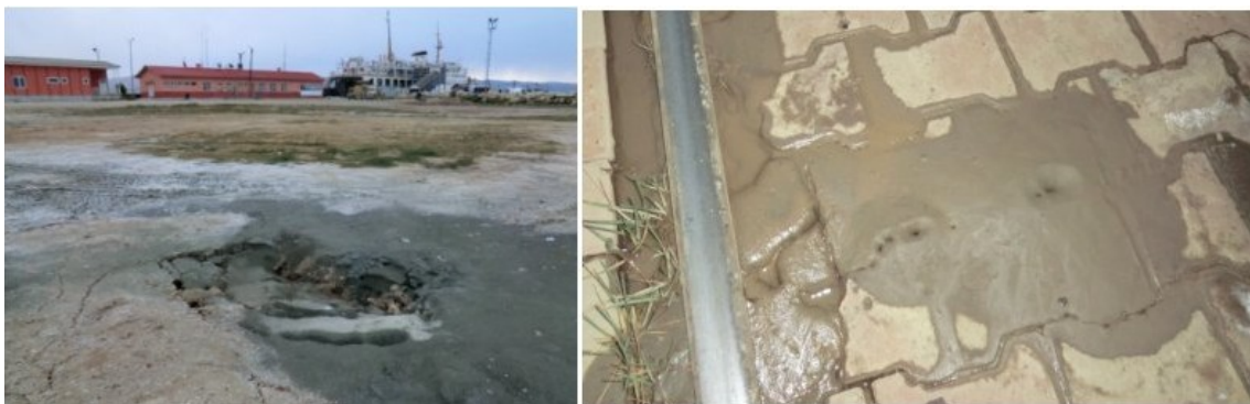
Figure 8.10. Views of deformed railways and liquefaction at Van Port.
