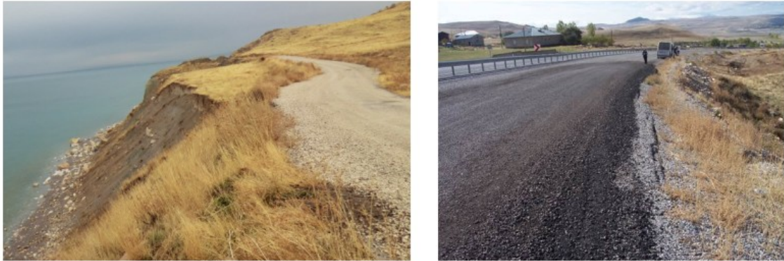
Figure 8.3. Failure of shoulder embankment of roadway and D975 Van-Ağrı Highway.
