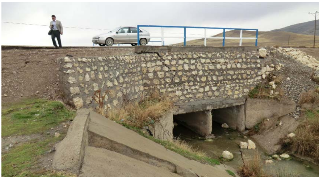
Figure 8.6 Damage to a bridge near Göllü village due to lateral spreading.
