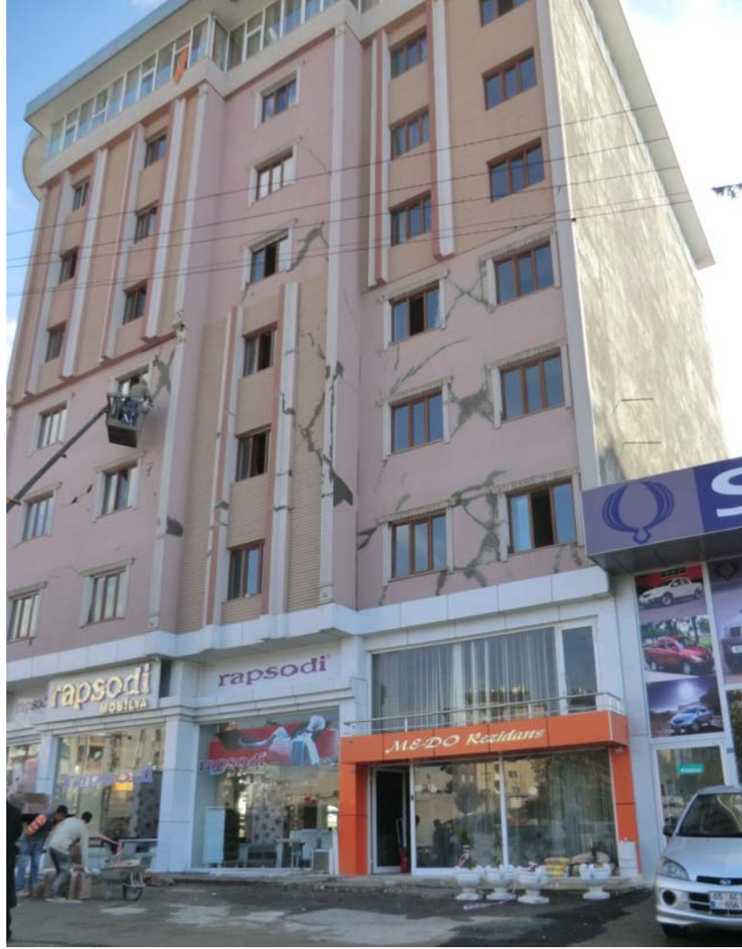
Figure 11.12. Cosmetic repairs applied to a damaged RC building in Van on November 5, 2011 after the Van-Erciş earthquake.
