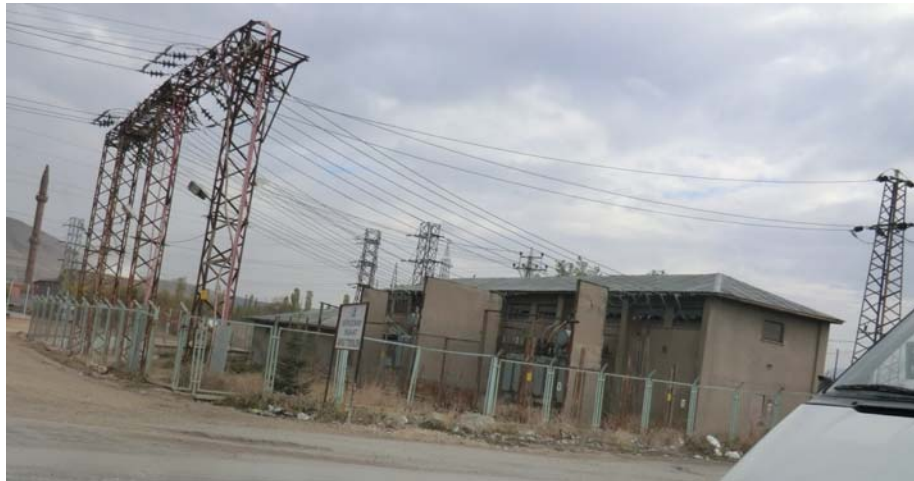
Figure 9.4. A non-damaged sub-station in Van.
