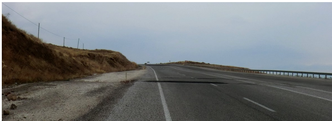
Figure 8.2. Embankment failure on the D975 Van-Ağrı Highway
