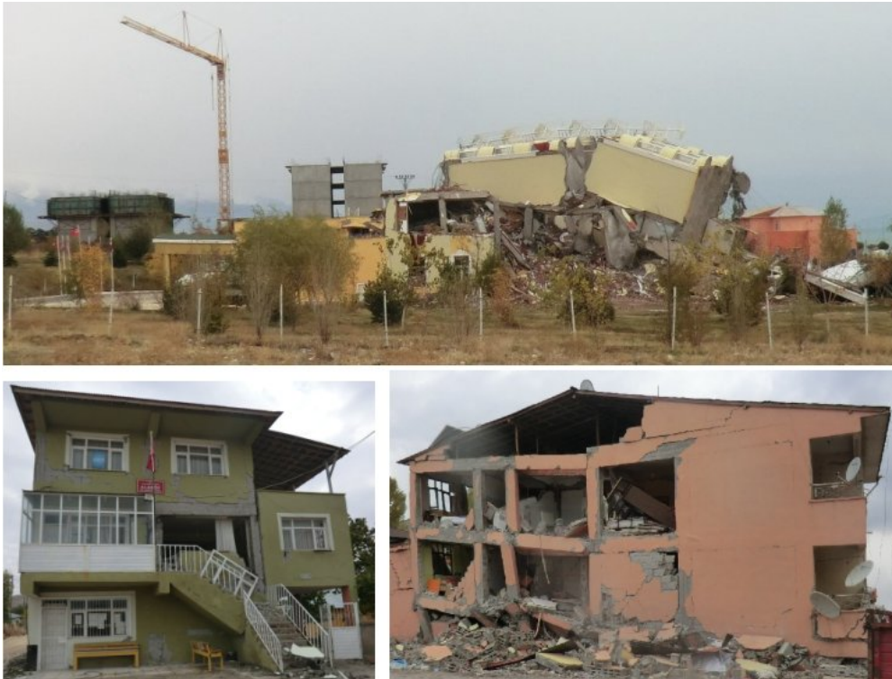
Figure 7.2. Views of collapsed or heavily damaged RC buildings.
