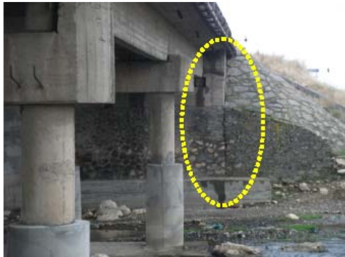
Figure 10.17. Crack and settlement on the right abutment of the bridge on the İrşat Stream between Erciş and Adilcevaz indicate due to liquefaction.
