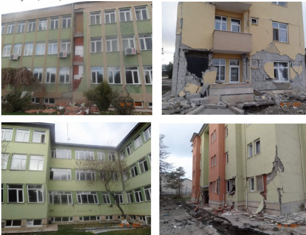
Figure 11.11. Views of heavily damaged reinforced concrete buildings of DSI in Van (Van-Edremit earthquake) (Photos: Ayhan Koçbay).
