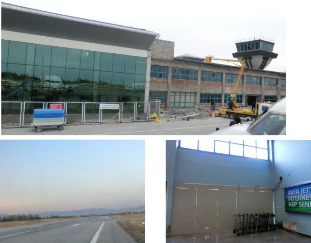
Figure 8.14. Views of runway and old and new terminal buildings of Van Airport suffered slight damage (note that the façade of the old terminal building thorn down before earthquake).
