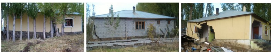
Figure 7.8 Lateral spreading induced damage to buildings in Çelebibağı village (Erçiş).
