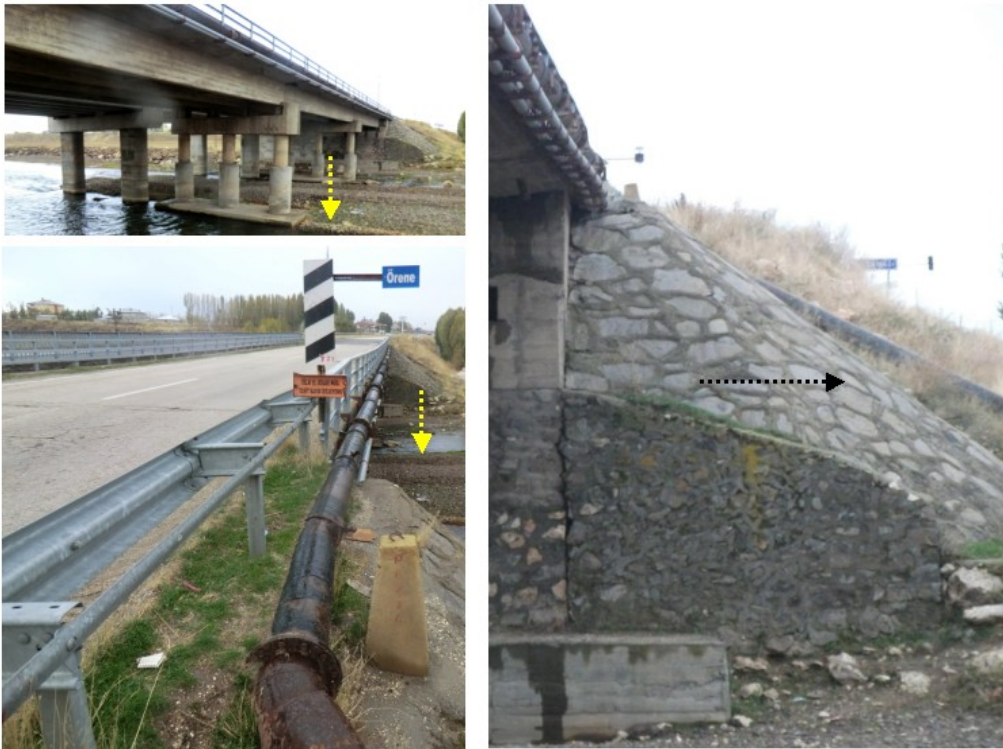
Figure 8.7. Settlement of piers and lateral deformation of embankments of Zilan Bridge.
