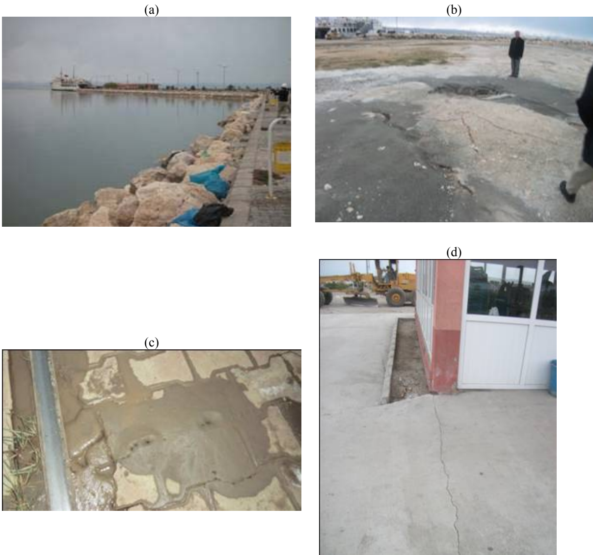
Figure 10.12. (a) A view from Van port, (b) liquefaction fissures and sand boils, (c) settled station building and (d) ejected sand along the contacts of pavement stones between rails (Van Port).
