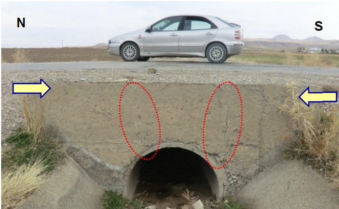
Figure 8.9. Cracking of wing-walls of a small bridge due to ground deformation caused by the thrust faulting.
