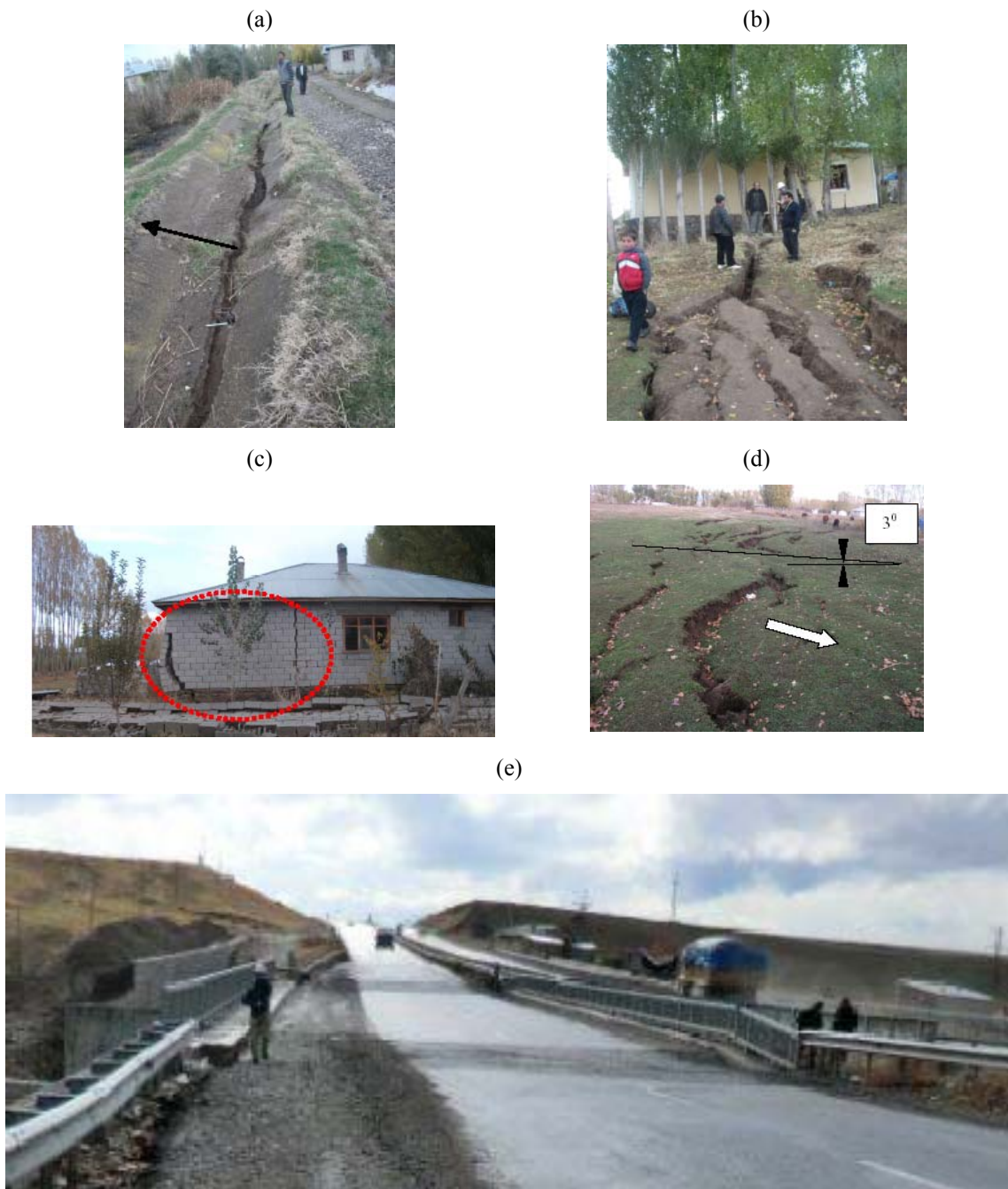
Figure 10.24. Lateral spread and resulted damages in Çelebibağ village: (a) damaged canal, (b-c) damaged residential houses and (d) movement and cracks due to lateral spreading, and (e) damage to piers and abutments of the Tirleşin Bridge due to settlement and lateral spreading of ground.
