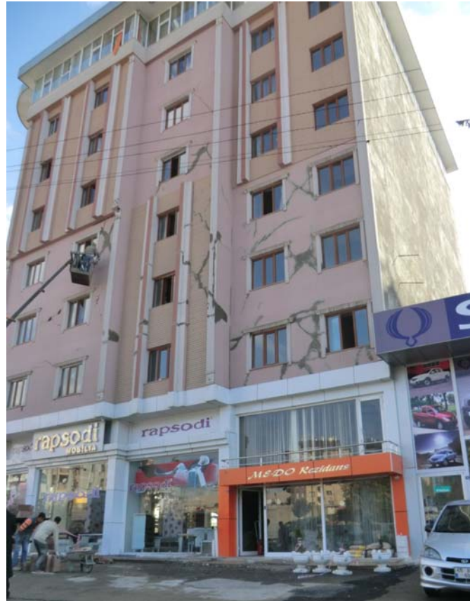
Figure 7.5. Cosmetic repairs applied to a damaged RC building in Van on November 5, 2011 after the Van-Erciş earthquake.
