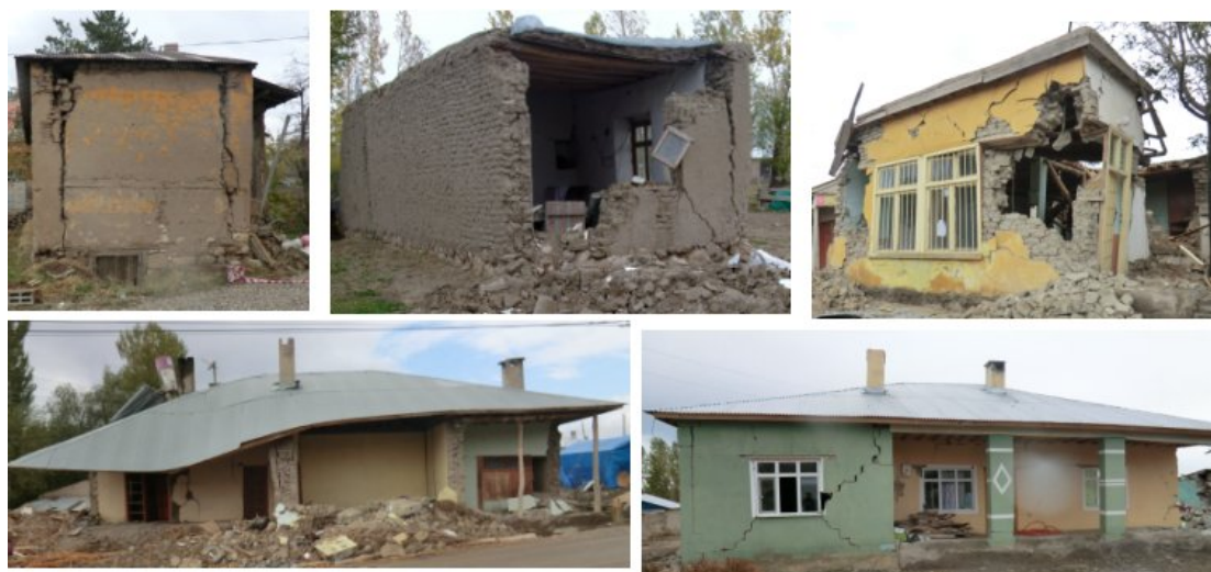
Figure 7.7. Views of heavily damaged brick masonry buildings.
