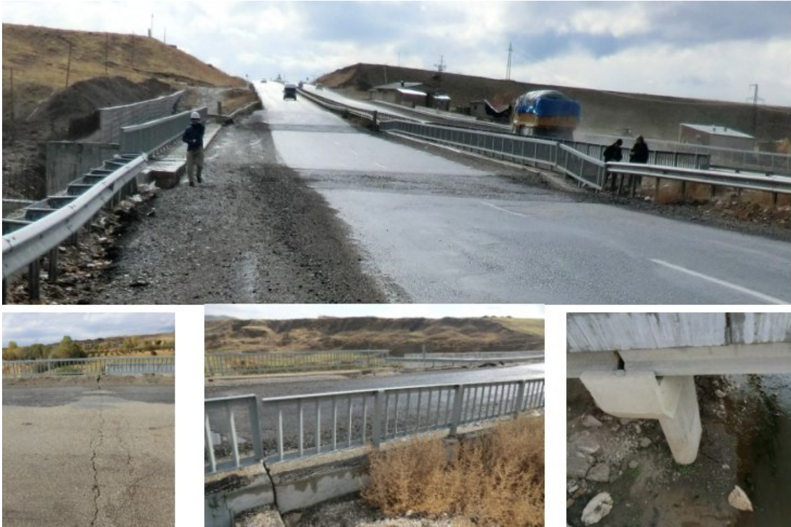
Figure 8.5. Views of damaged Tırleşin bridge over Karasu on Van-Ağrı Highway.
