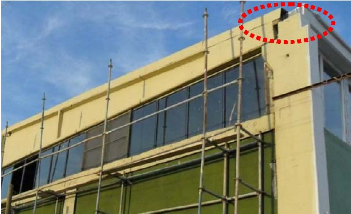
Figure 7.13. A typical damage to a pre-cast reinforced concrete structure in Van Industrial Complex (from KOERI, 2011).
