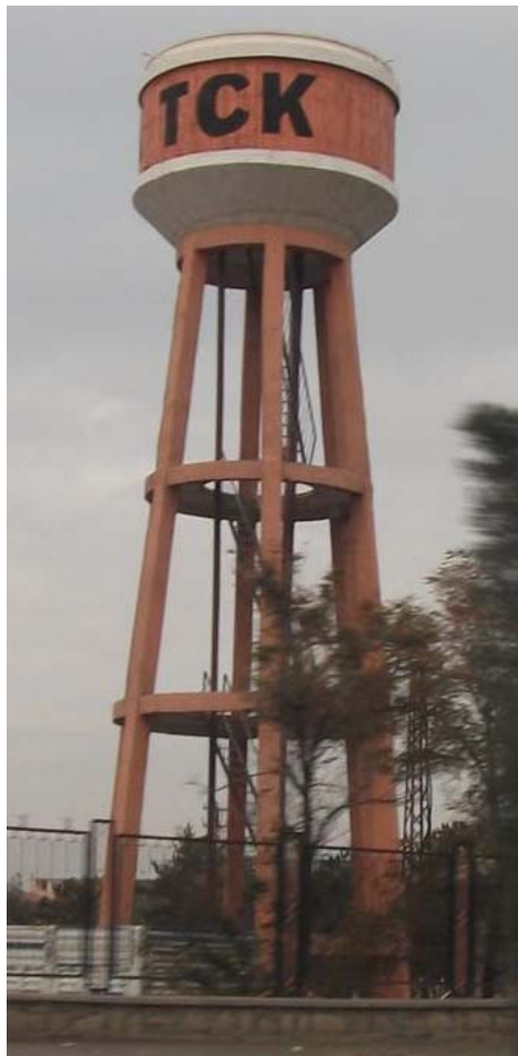
Figure 7.10. Non damaged elevated water tank owned by the General Directorate of Highways (TCK) in Van city.
