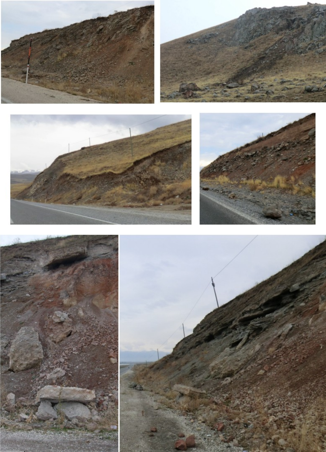
Figure 8.4. Slope instabilities and rock falls along Van-Ağrı Highway.
