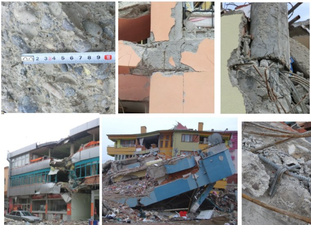
Figure 7.3. Views of constructional problems causing the collapse or heavy damage.
