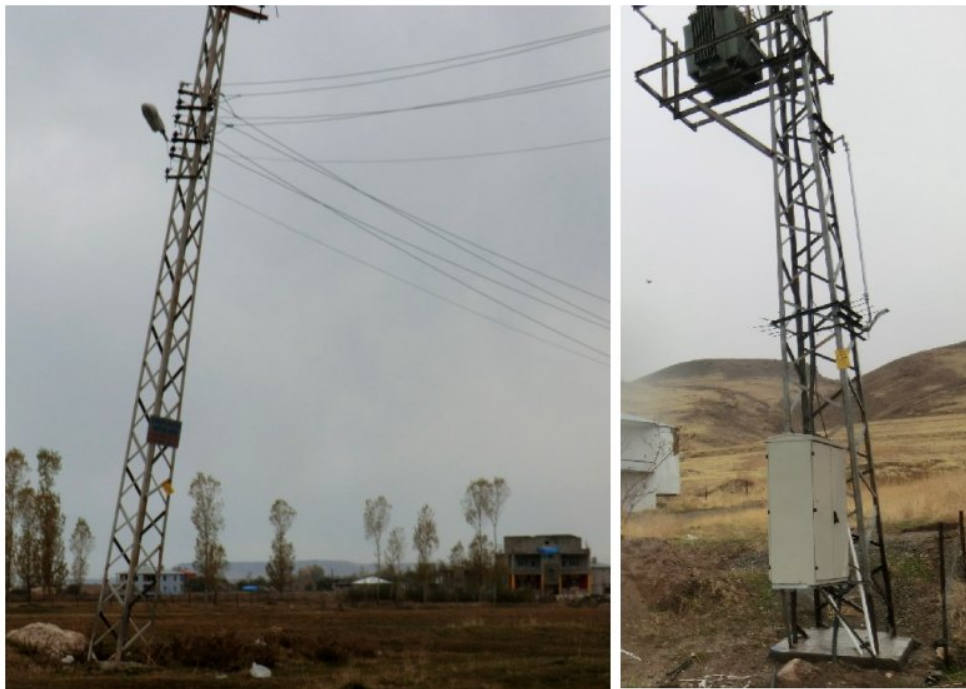
Figure 9.7. Tilted and bended utility poles in Van and Yeşilsu.
