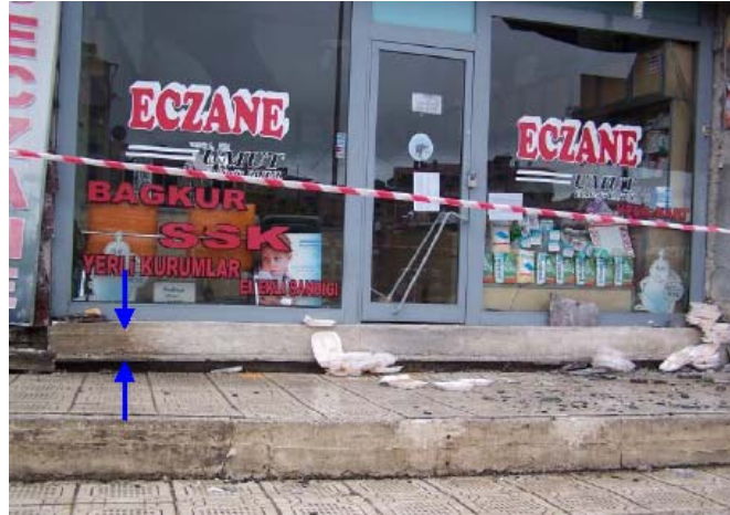
Figure 10.18. Settlement of a building probably due to liquefaction in Erciş town (after JMO, 2011).
