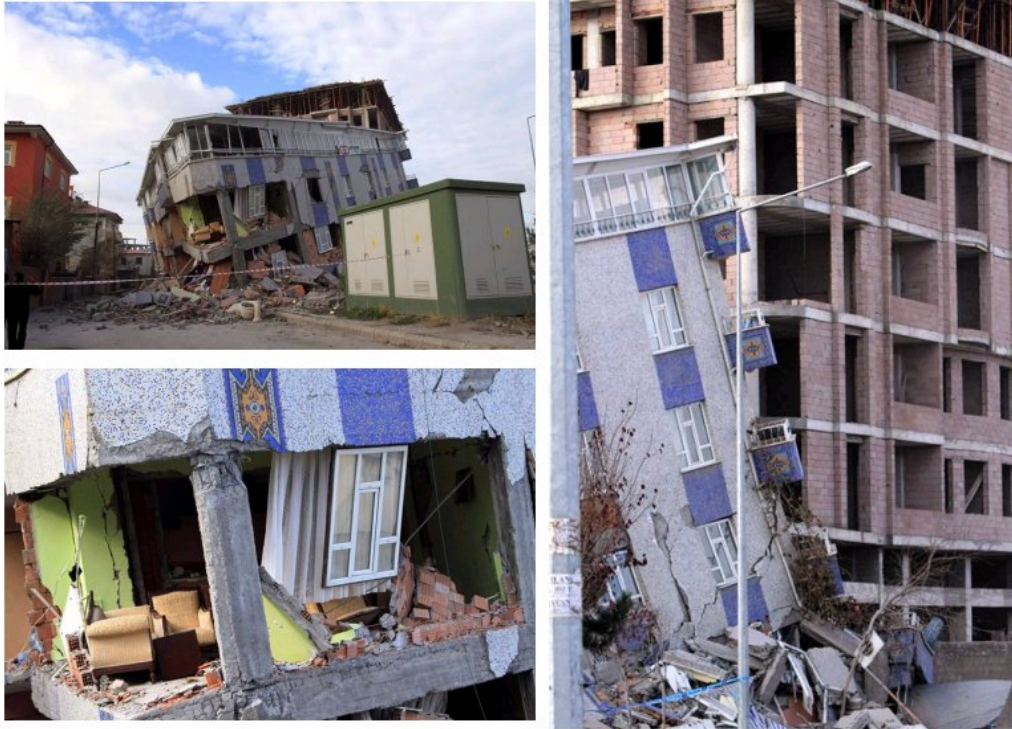
Figure 11.10. Views of a collapsed reinforced concrete building in Van (Van-Edremit earthquake) (Anadolu Ajansı, 2011).
